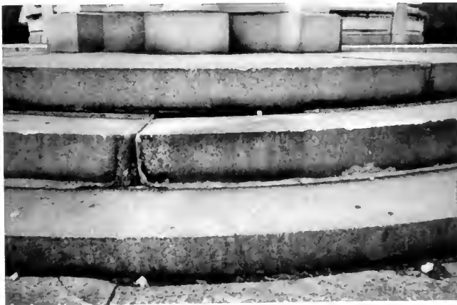
Figure 40: Granite base with open joints and misalignment of masonry units
